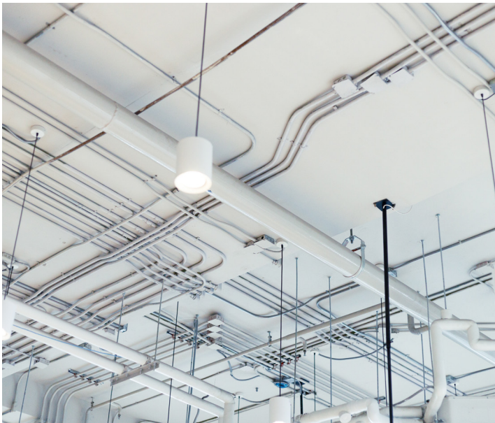
Multiple runs of conduit overlaid and hardwired to a factory ceiling
